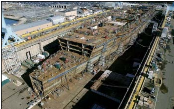
A view of the construction of George H.W. Bush (CVN 77) as of Dec. 8, 2004. The ship is scheduled to be launched in October of 2006. Photo by Chris Oxley
