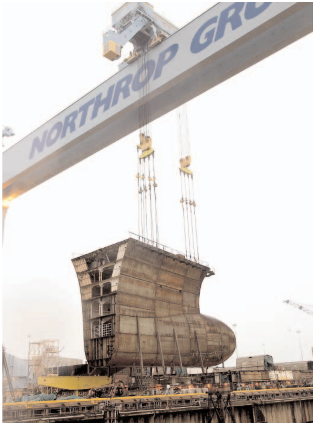
Newport News' 900-ton crane begins lifting the lower bow unit of George H.W. Bush (CVN 77) on March 8. Photo by Chris Oxley
